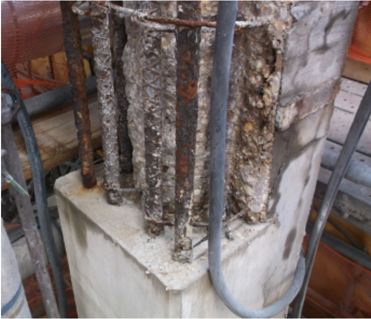
Reinforce Concrete Deterioration
