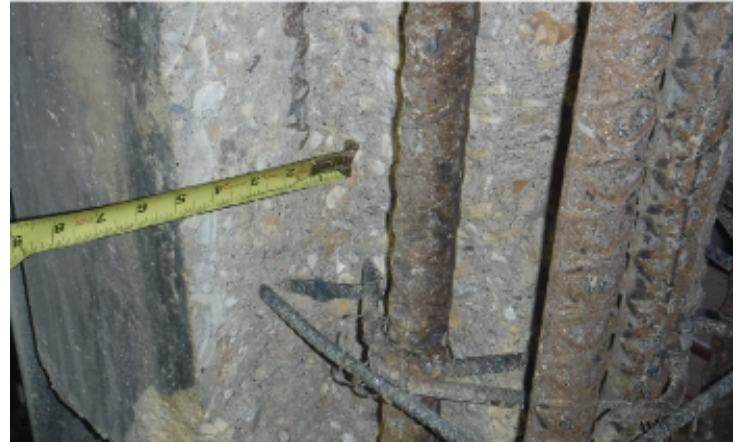
Reinforce Concrete Deterioration 5"
