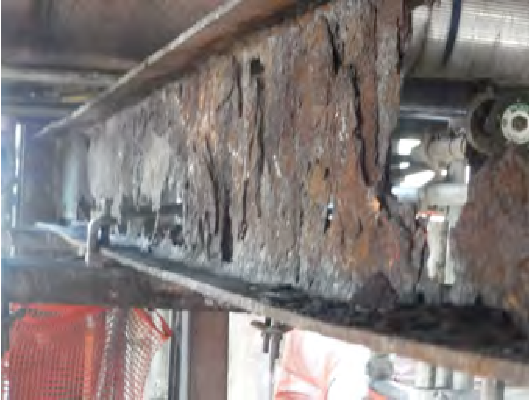
High Risk Steel Defect
