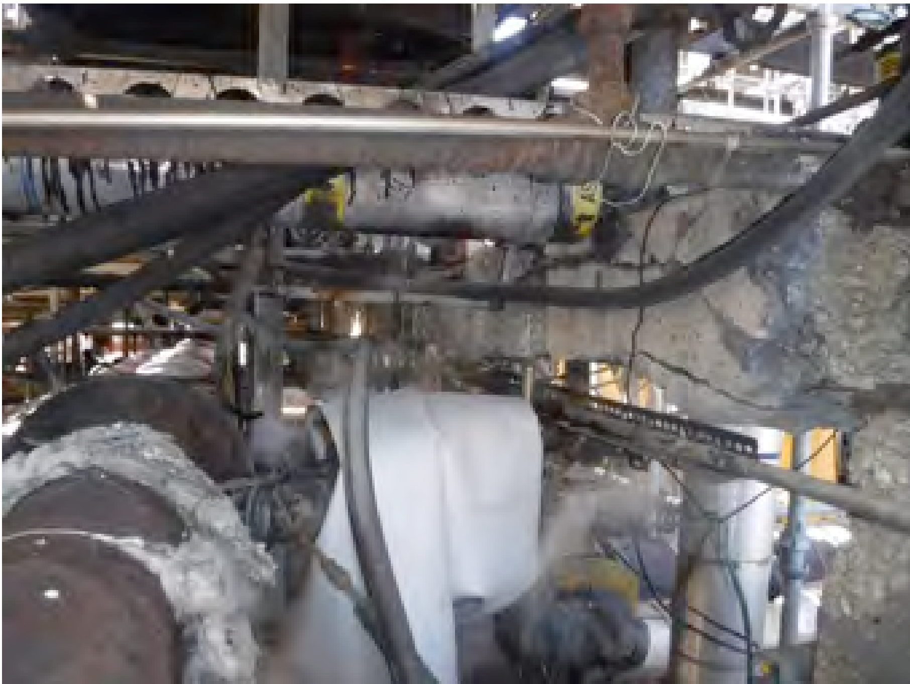
High Risk Concrete Defect
