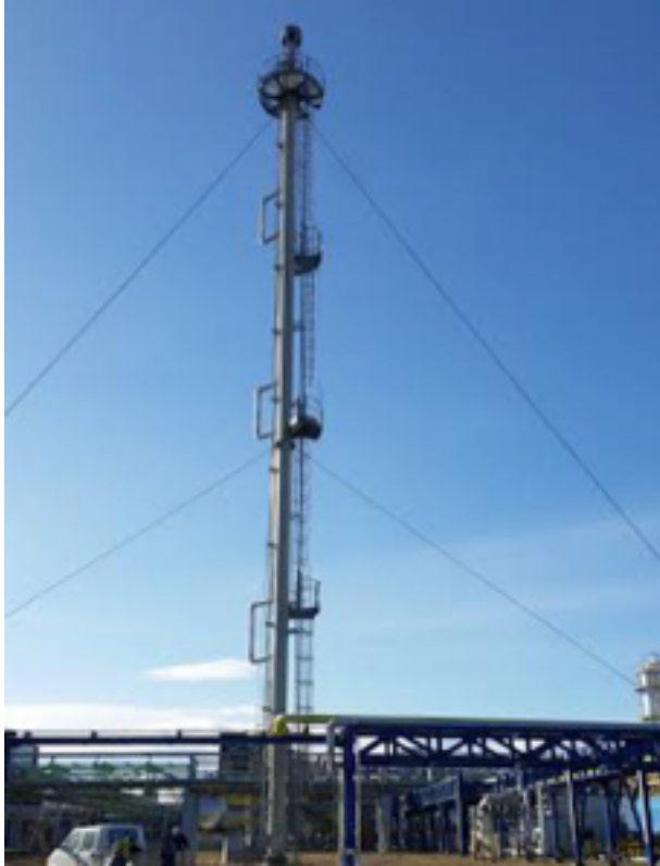
Typical Guyed Flare Tower
