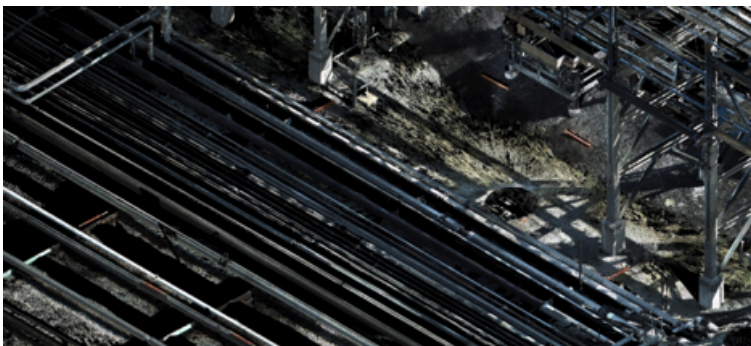
3D Point Cloud Scan of Pipe Alley Prior to Piping Model Creation
